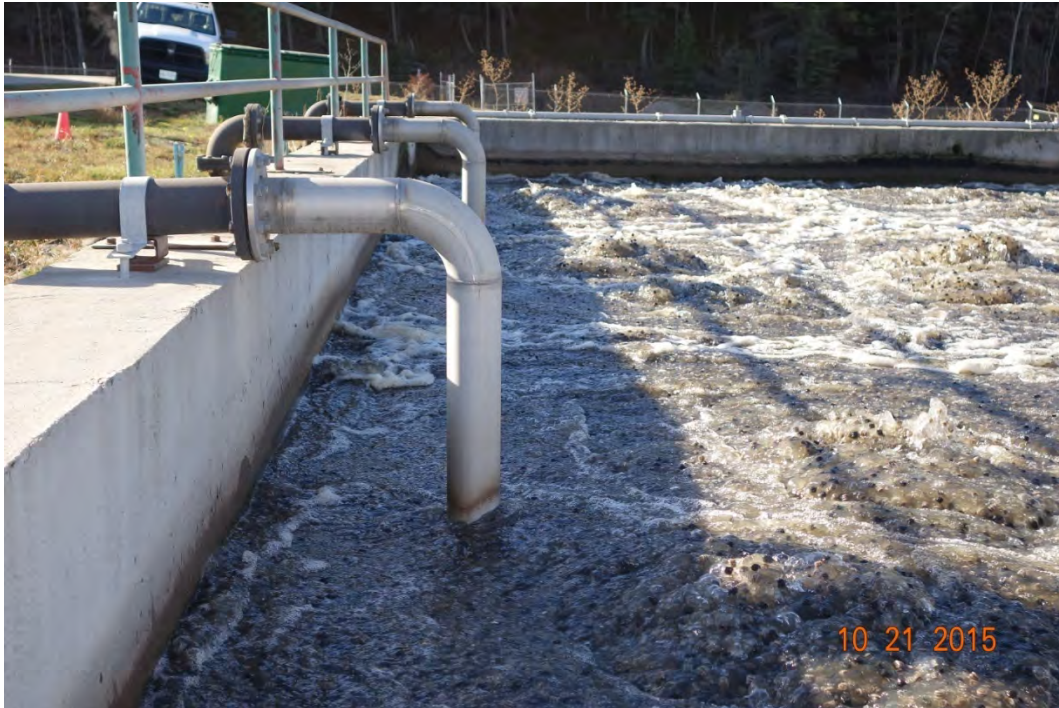
FIGURE 4-7: MBBR TANK AT RADIUM HOT SPRINGS WWTP (HIGHLIGHTED)
