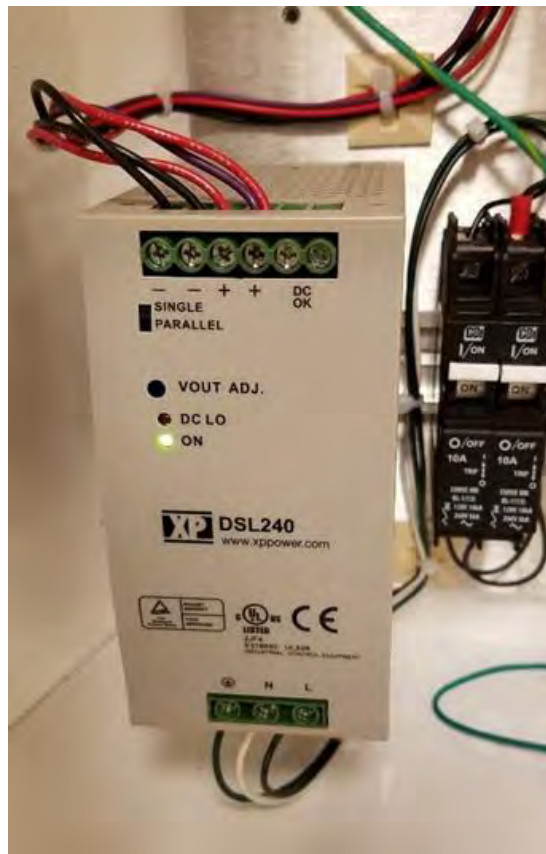
Figure 10 - Power Supply Mounted and Wired
